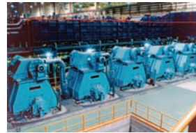
Main Motors Metal Rolling Mill
